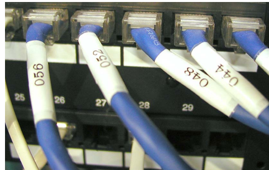
Figure 1. Cables Labeled by Numbers
